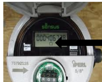
Leak Indicator: Circle in center under the numbers (Water movement is noted by a positive symbol (+). If a negative symbol (-) is present, water is moving backwards through the meter, known as "backflow".)
