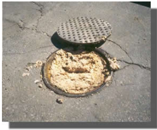
Fact: Fats, oils, and grease originating from food preparation clog sewer lines. Source: City of Virginia Beach (2008).
